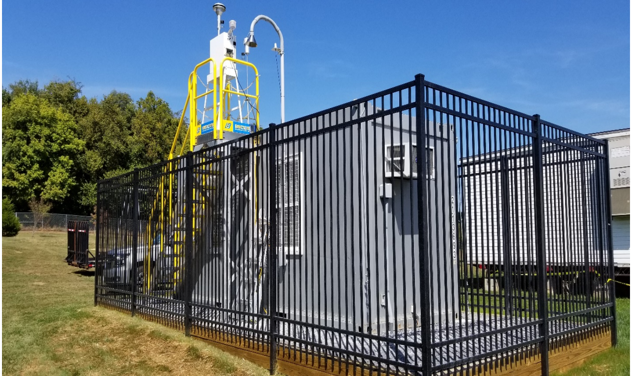
Figure 5: North Jefferson Elementary School Monitoring Location
